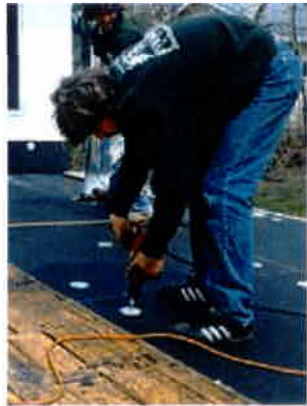
Figure 1. EPDM is installed over a special felt-covered insulation board. Screws and large metal fastener plates secure the insulation board to the roof deck.
