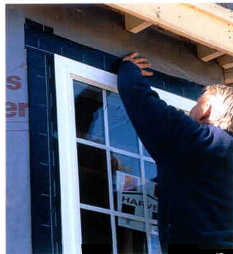
Roofing nails hold in vinyl windows. Here's about the only difference in installation: Vinyl is easily cracked by an errant hammer blow, particularly in the cold. Once the window is in, self-adhering flashing tape seals out water.
