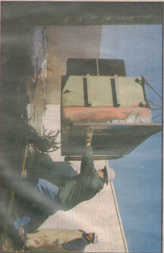
Ian Wingfield , Daily Herald Craig Pierce , with Utah Power, positions the burned out electrical transformer while it is hoisted up by a crane at Mountain View High School on Friday.
